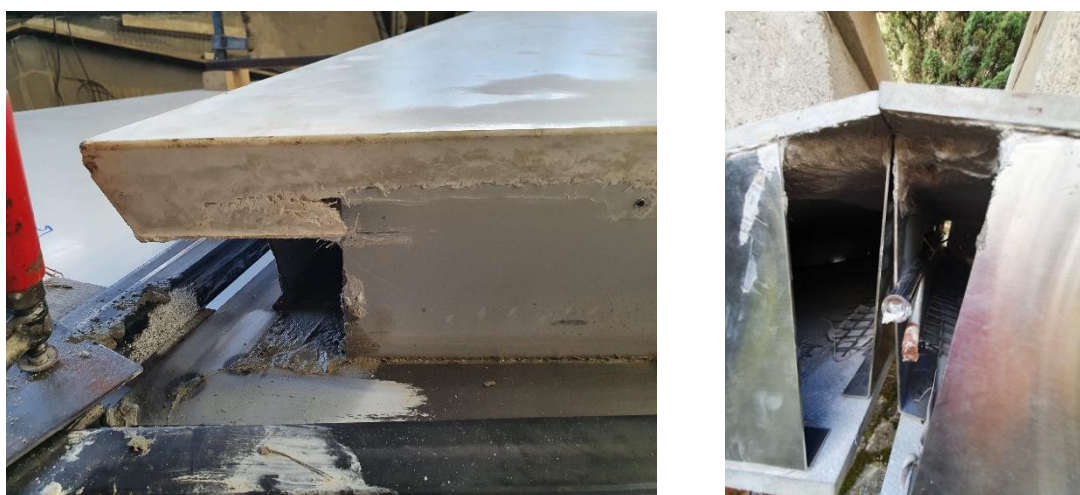
Figure 2: Inaccuracy in steel-to-concrete connections and joint misalignment causing non-shear behavior of the structure.
